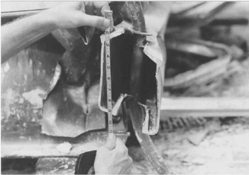
EXHIBIT 2.3 Fourth-floor box beam showing a hole where it pulled free from the ceiling suspension rod. The hanger rod to the second floor is still in place.
